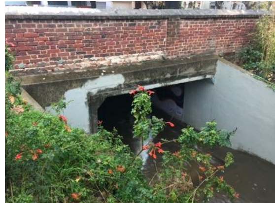
Huge concrete culvert installed under Osmond Terrace and William Street by the NP&StP Council.
